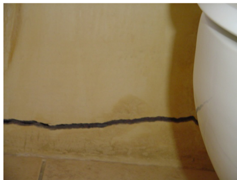
Figure 4-27 Severe floor settlement
