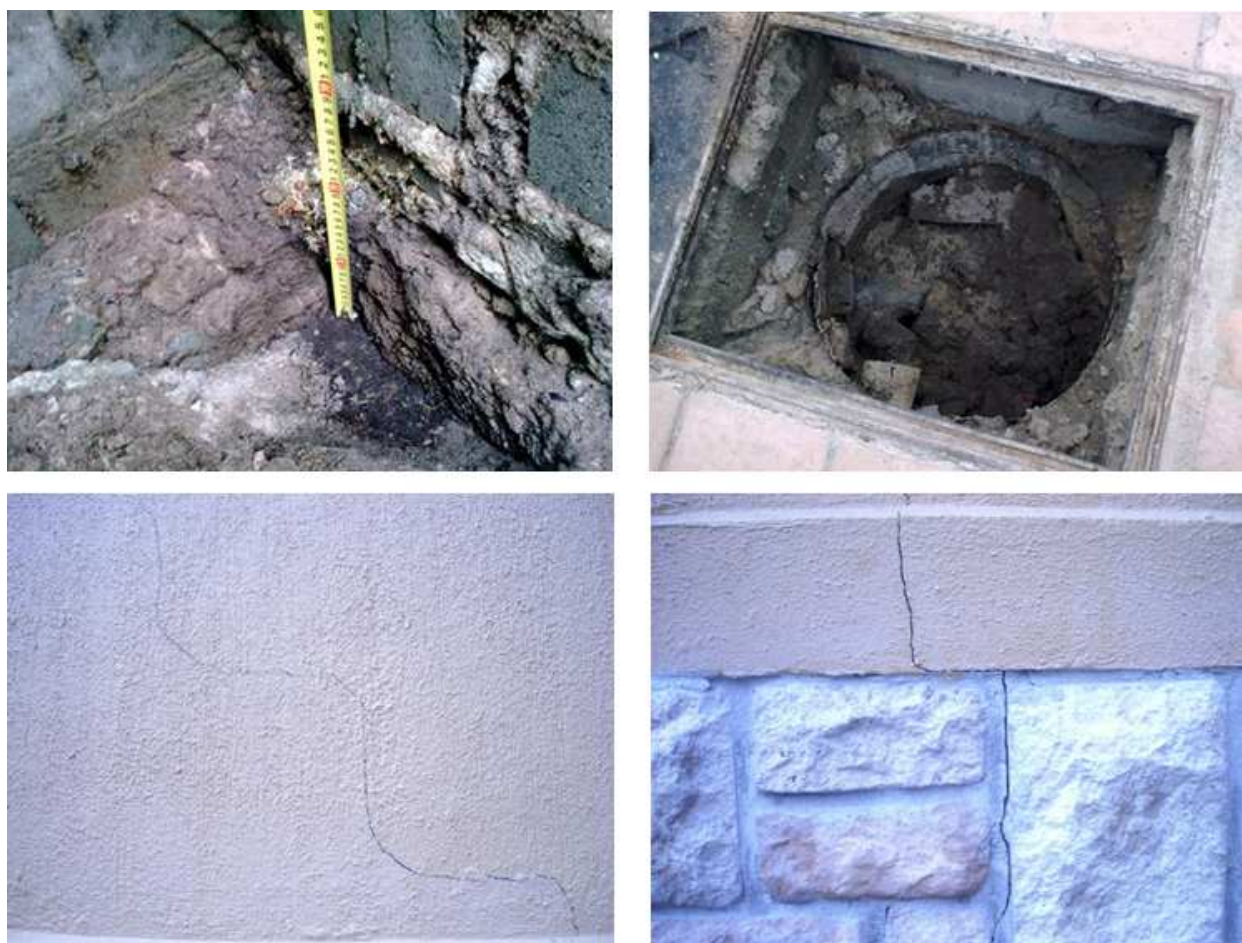
Figure 3-26 Images of light structural damage and poor drainage
