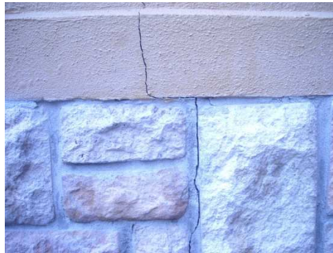
Figure 4-26 Light settlement cracks
