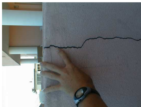
Figure 4-28 Moderate settlement cracks
