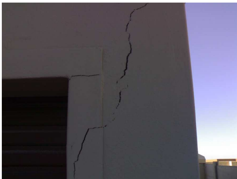
Figure C.2 NHBRC images of severe vertical settlement cracks
