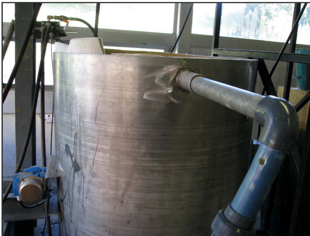
Figure 3-4 Water overflow drain
