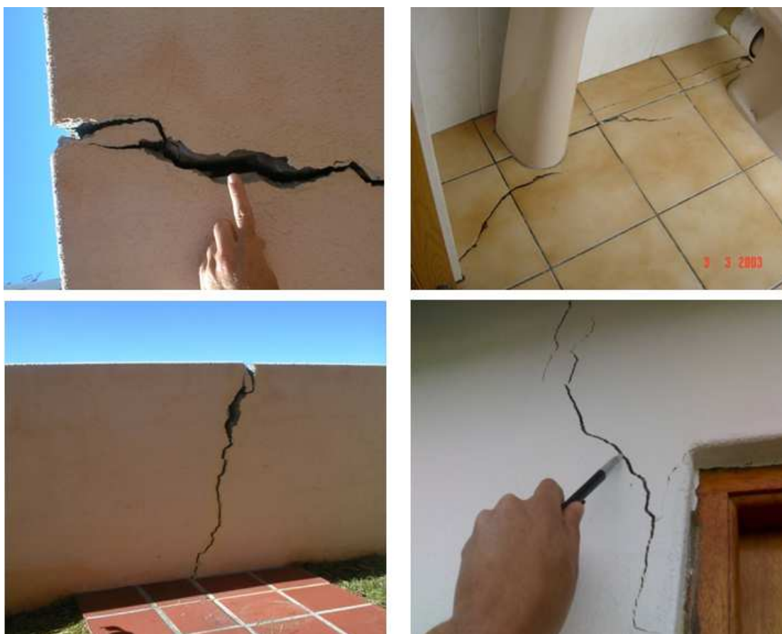
Figure 3-25 Images of structural damage (Courtesy NHBRC, 2003)
