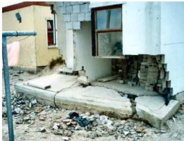
Figure 2-10 Erosional collapse (Goliger, et al, 2008)
