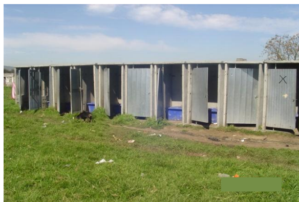
Figure 3-5: Dry sanitation type container toilet
