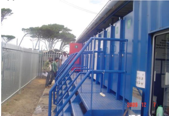
D1: MobiSan facility installed at Pooke se Bos Informal settlement (Cape Town)
