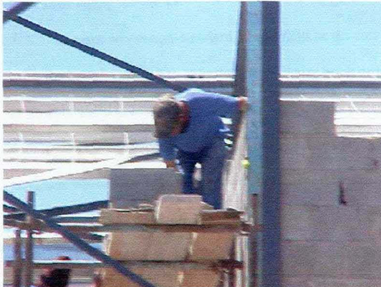
Figure 4.1: Bricklaying artisan bending to scoop mortar placed at his feet on the scaffold.
