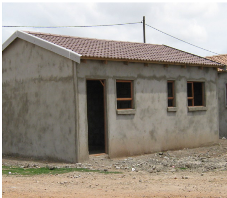
Fig. 3 represents the plaster work that has been done on the house. The plaster mix is a 1:4 plaster mix.
