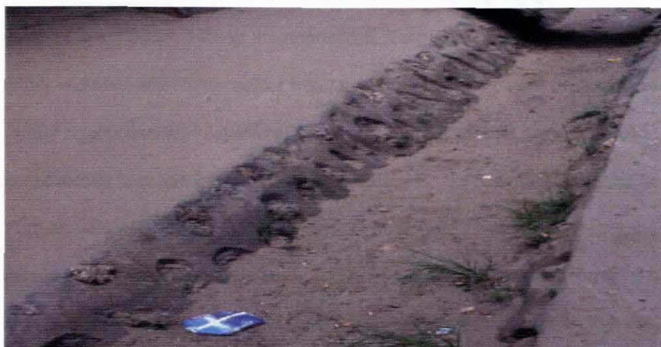
Figure 5.14: Surface water drain in the Mabatini settlement, February 2005
