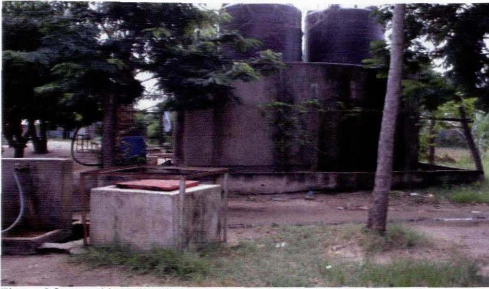
Figure 5.21: Potable well with two storage tanks in Tabata, February 2005
