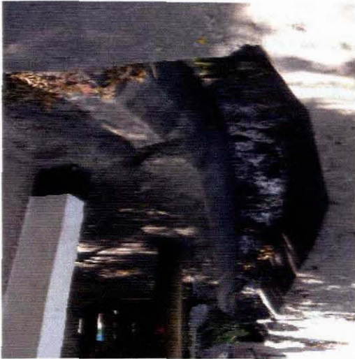
Figure 5.3: Side drain in Hanna Nassif, January 2005.
