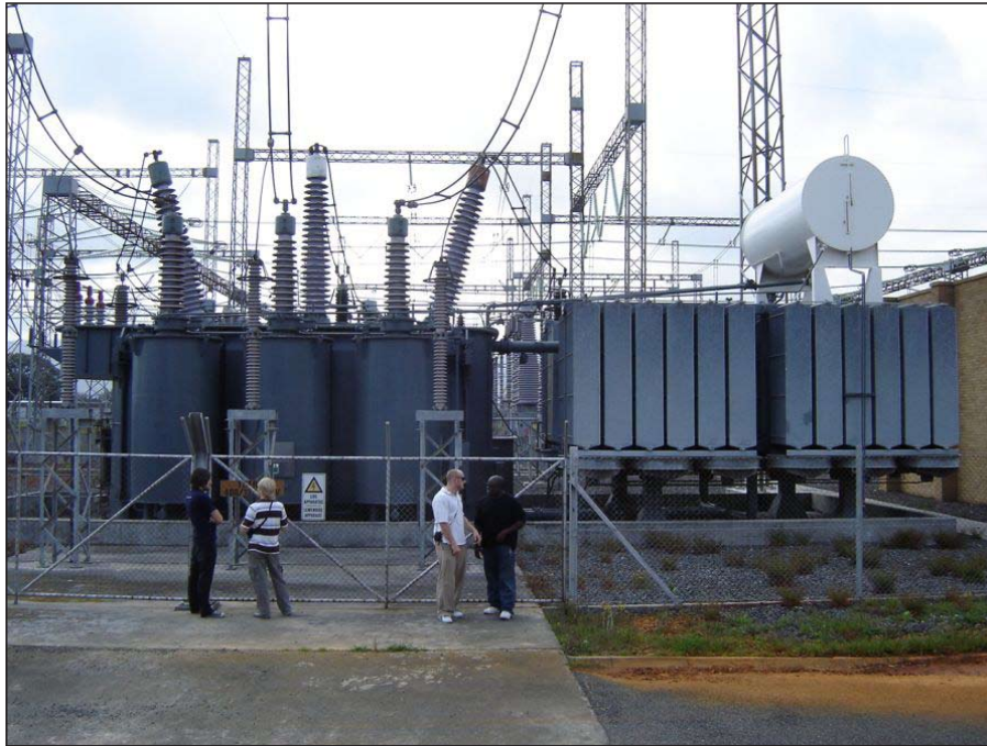
Figure 4.2: 500MVA power transformer
