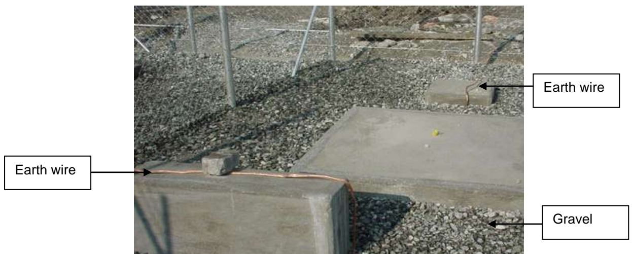
Figure 5.2: Earth wires at harmonic filter site
