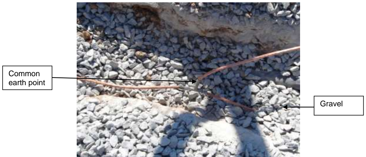
Figure 5.3: Common earth point at harmonic filter site
