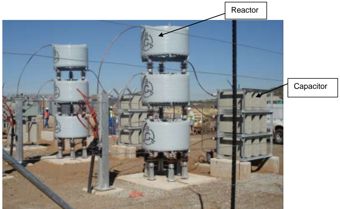
Figure 6.19: Series tuned harmonic filter at site
