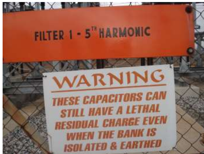
Figure 5.6: Warning sign at the fence of harmonic filter site
