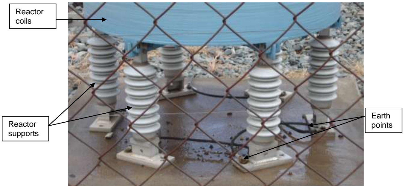
Figure 5.17: Reactor supports earthed
