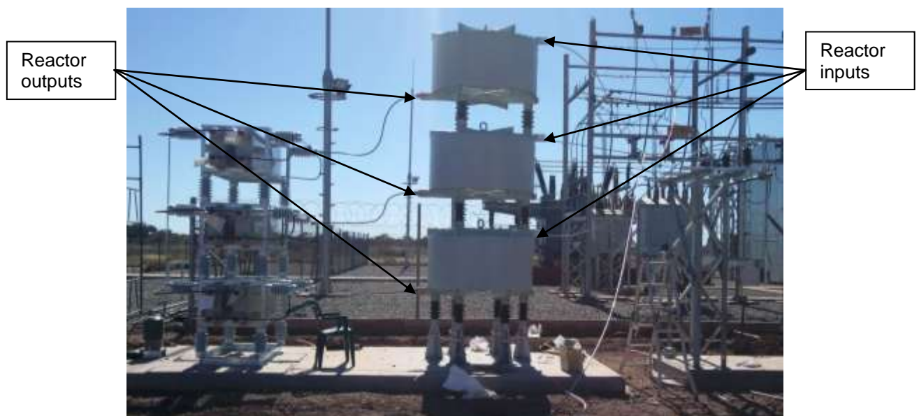
Figure 5.15: Reactors electrical input and output connections
