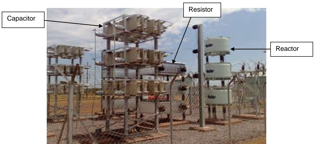
Figure 6.28: Second order harmonic layout after installation.
