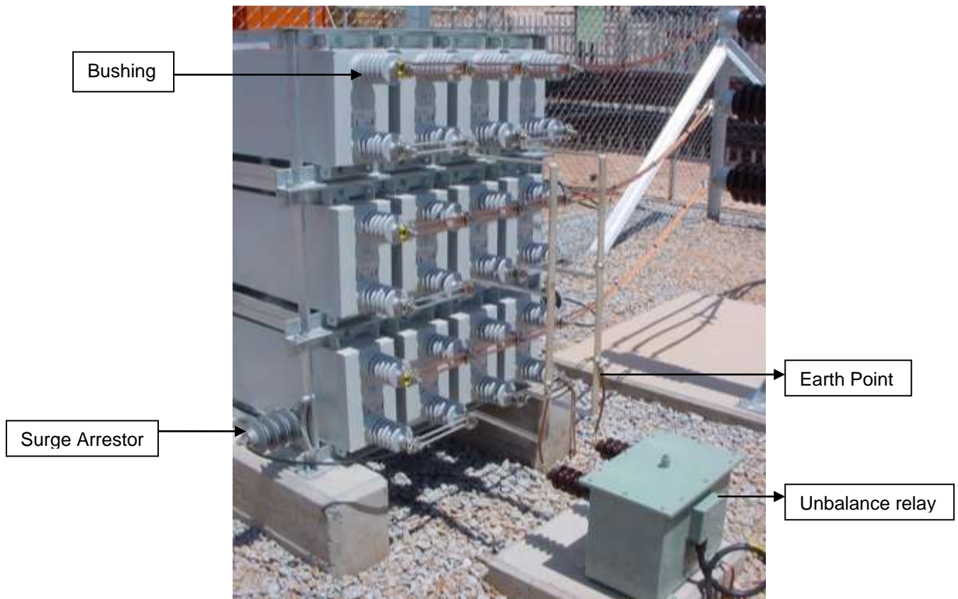
Figure 5.12: Unbalance relay and surge arrestor connected to capacitor banks
