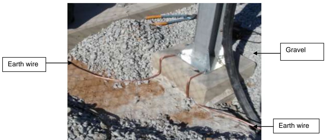
Figure 5.4: Earth points connection at harmonic filter site
