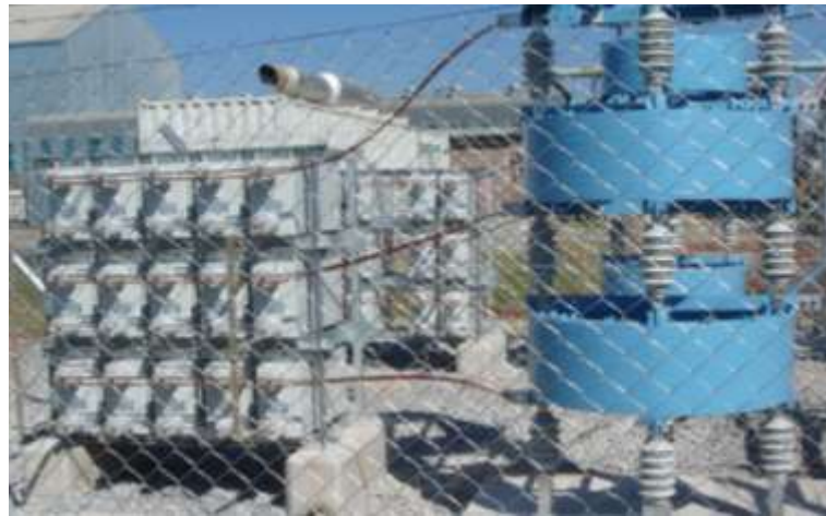
Figure 2.1: Series tuned harmonic filter at site
