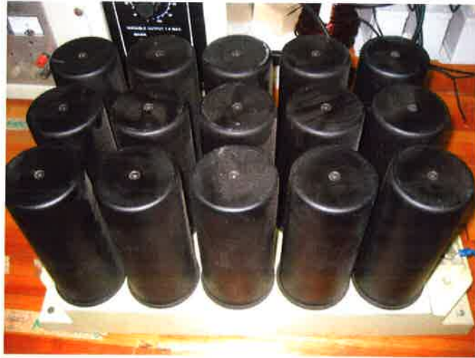
Figure 6.12 Dc link bulk Capacitors
