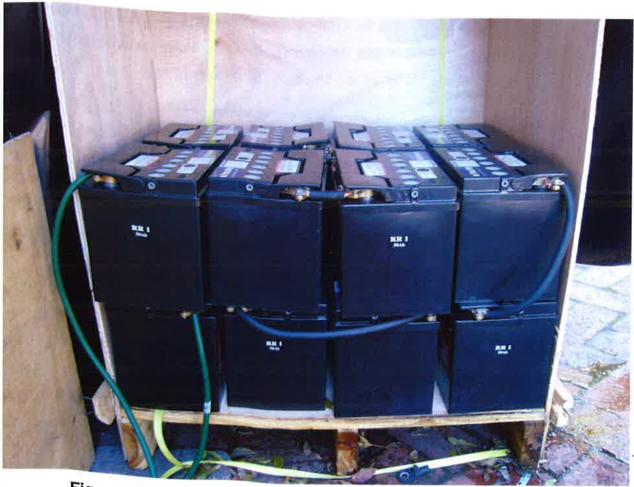
Figure 6.9 196V Battery Bank as Supplementary Energy Supplies
