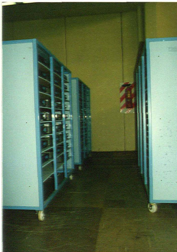
Fig 3-1-5 Photographs showing decoder soaking area. Every unit must be switched on for a minimum of 12 hours before final C.A.
