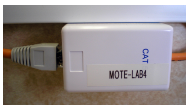
Figure A.2: Testbed network cable adapter box
