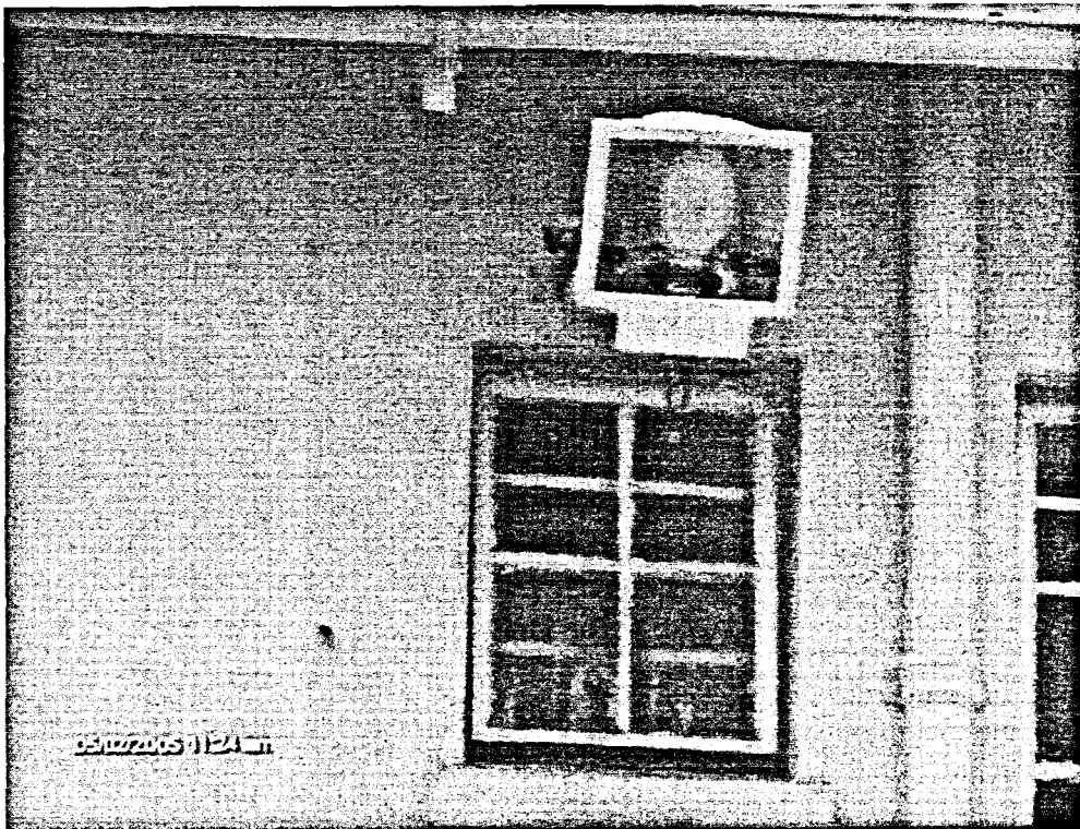
Figure 3.5.4: Various lamps and lamp-fittings installed on the premises (cont...)
