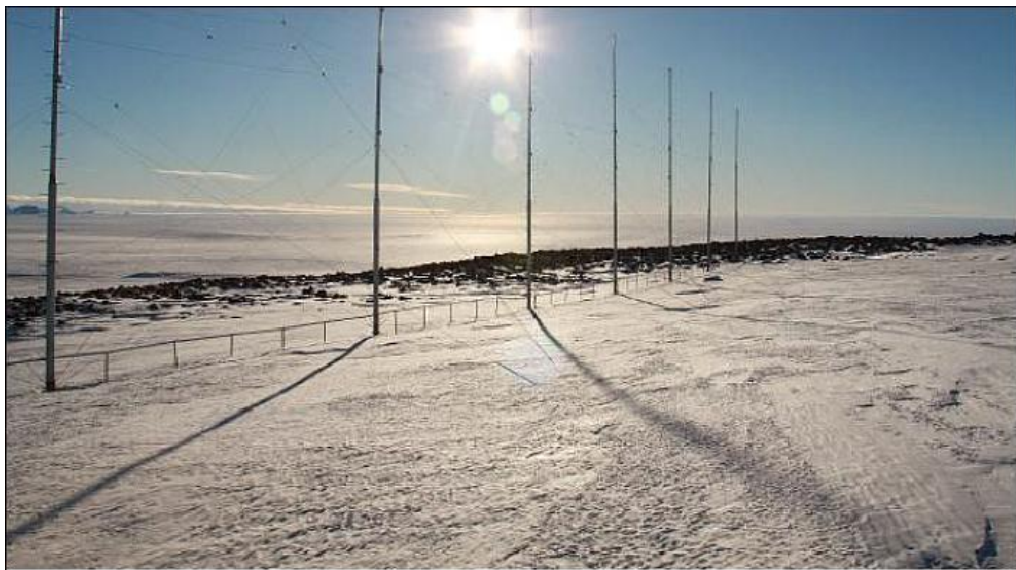
Figure 1-2: The 16-element Twin Terminated Folded Dipole (TTFD) antenna array of the SuperDARN radar in Antarctica (Adapted from Cilliers et al. , 2013:1290)
