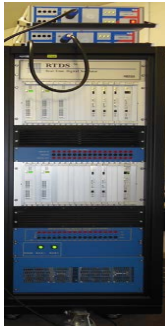
Figure 4.2: Real-Time Digital Simulators (RTDS) in the Centre for Substation Automation and Energy Management Systems (CSAEMS)
