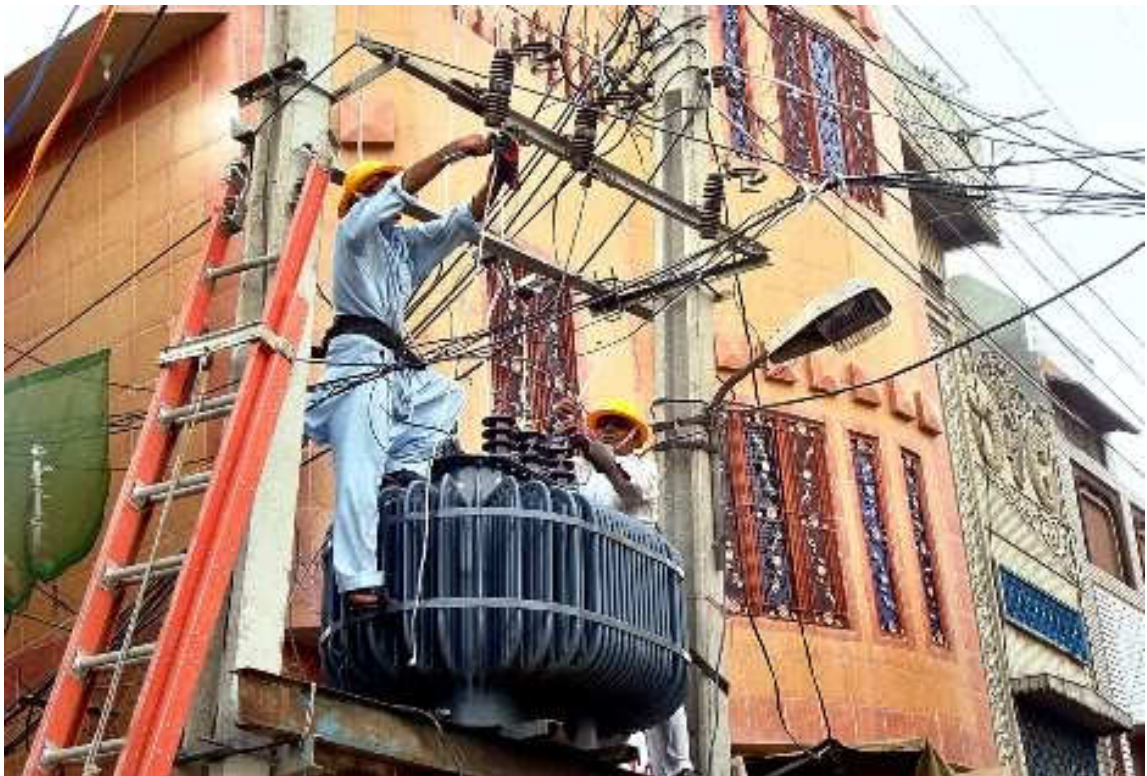
Figure 2-7 Utility worker performing routine transformer measurements (Mughal, 2008)
