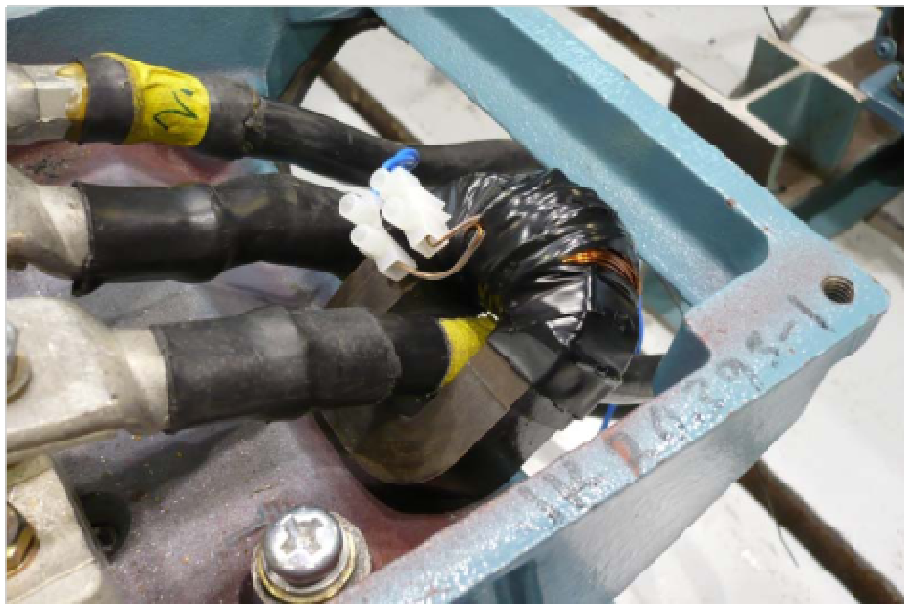
Figure 2-19CT clamped onto a motor phase conductor(Ahola, et al., 2008)
