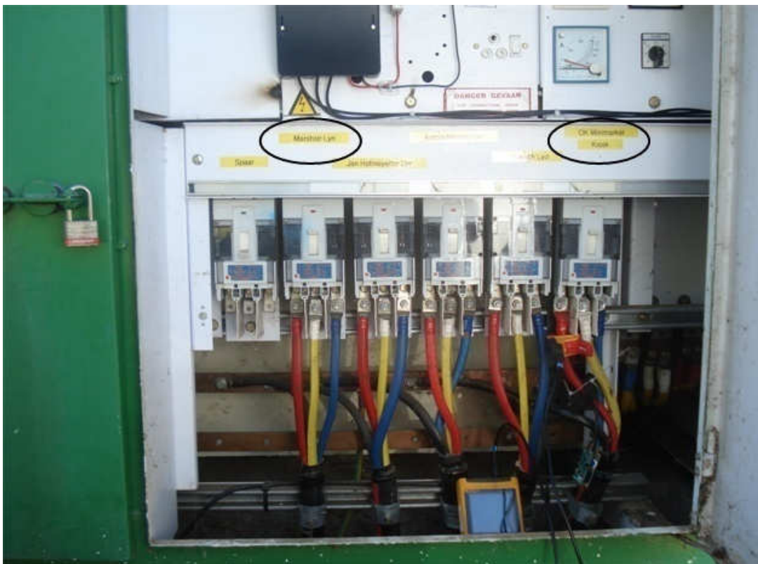
Figure 6-1 Internal layout of mini substation in Paarl
