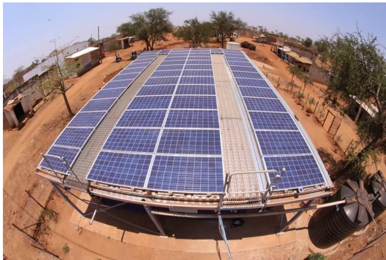
Figure 2.1: Makueni County 13.5 kW PV system, Kenya, Kitonyoni village market (Phys. Org, 2013)
