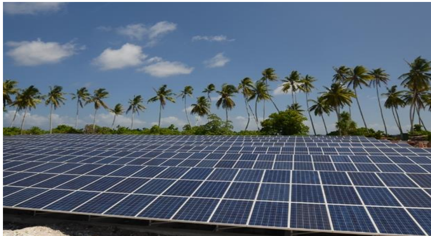
Figure 3.4: Solar panel array on Tokelau Island (Power Smart, 2012)
