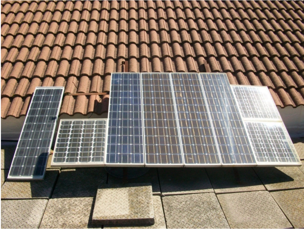
Figure 4-6: Solar panels mounted on the roof of electrical engineering department CPUT
