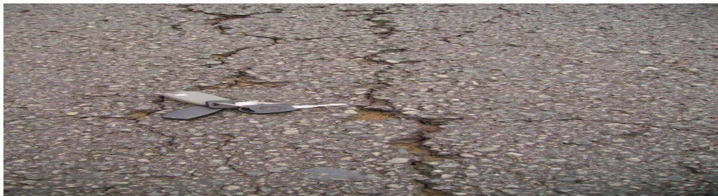
Figure 1: Cracked asphalt surfacing section. (Source: Own source)
