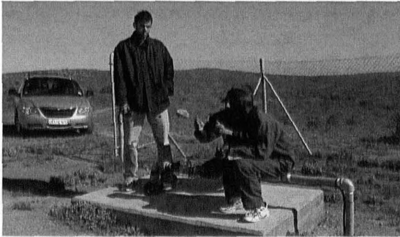
G5: Old configurations of flow & pressure transmitters
