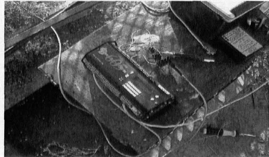
G12: Data logger, charge controller & a battery
