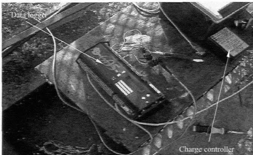
Figure 4.10: A data logger and a charge controller
