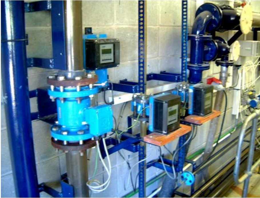
Figure D.2c Krohne in- line magnetic flow meters used in the 80 mm, 28 mm and 13 mm diameter PVC tubes.
