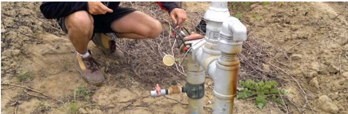
Photo 2.14 : Altus opening one of the many valves located between the vineyard blocks.
