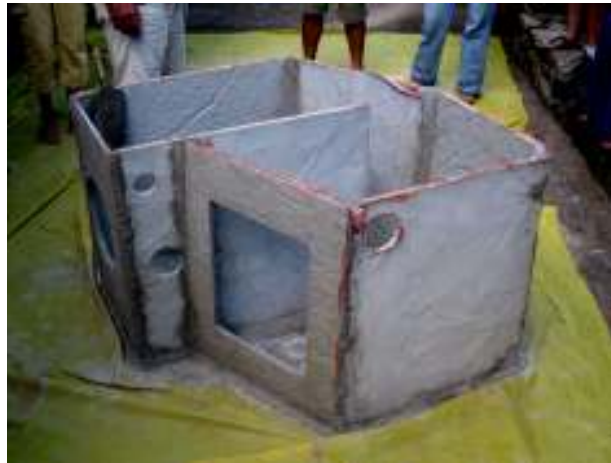
Fig 3.24 Dry Toilet being assembled from textile-reinforced cement panels (Photo: F. De Flamingh)
