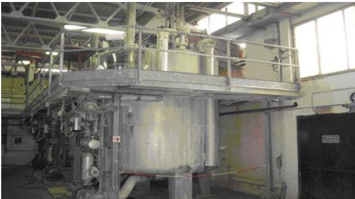
Figure 7.15: Fleshings storage tank (Source: Author's own, 2014)
