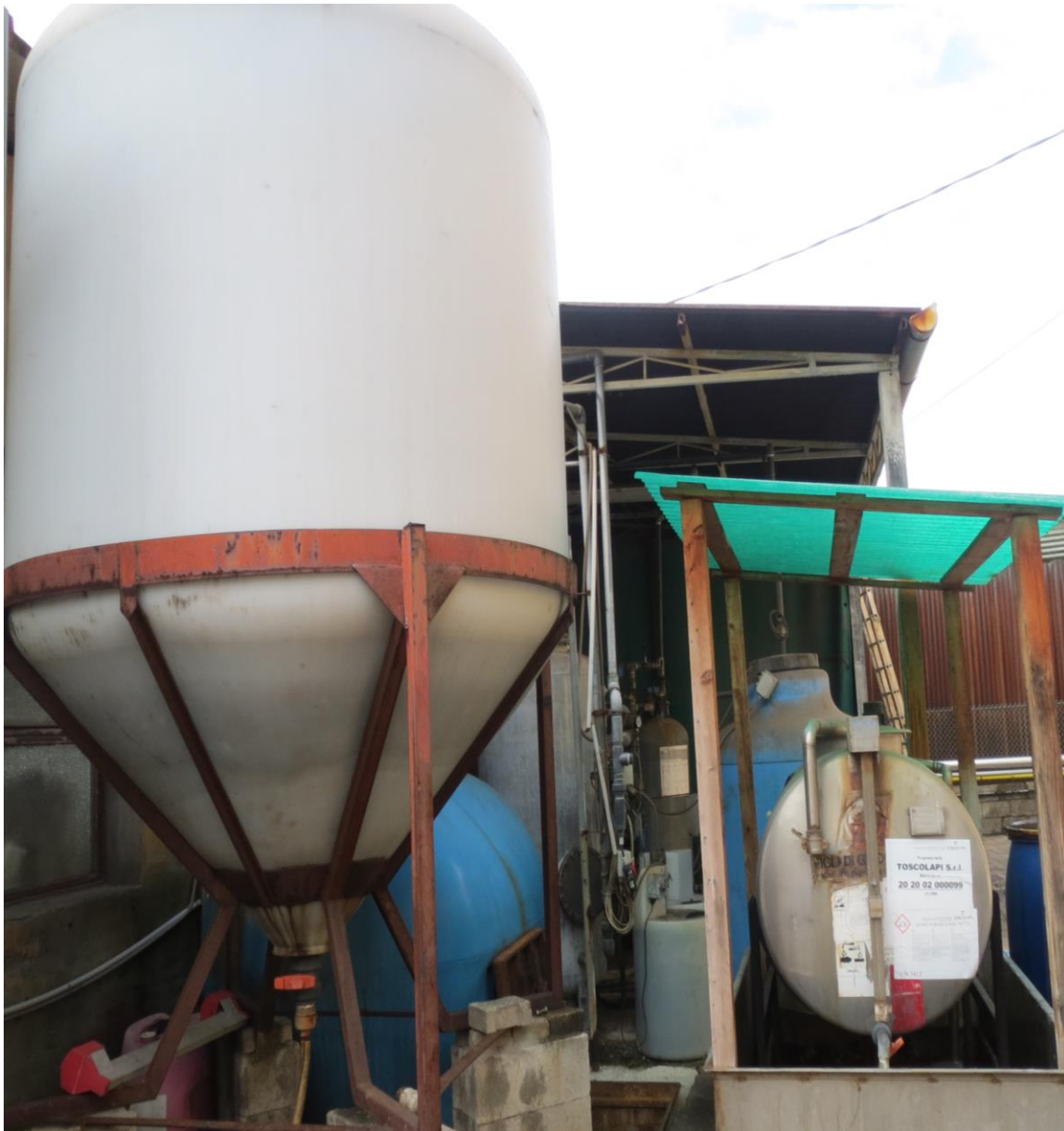
Figure 7.14: Wastewater receiver and meter pollution reading unit (Source: Author's own, 2013)
