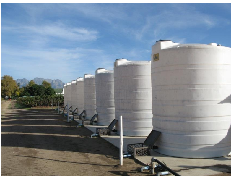
Figure 3.2. Wastewater mix and distribution plant in the experimental vineyard at the Goudini Winery at Rawsonville
