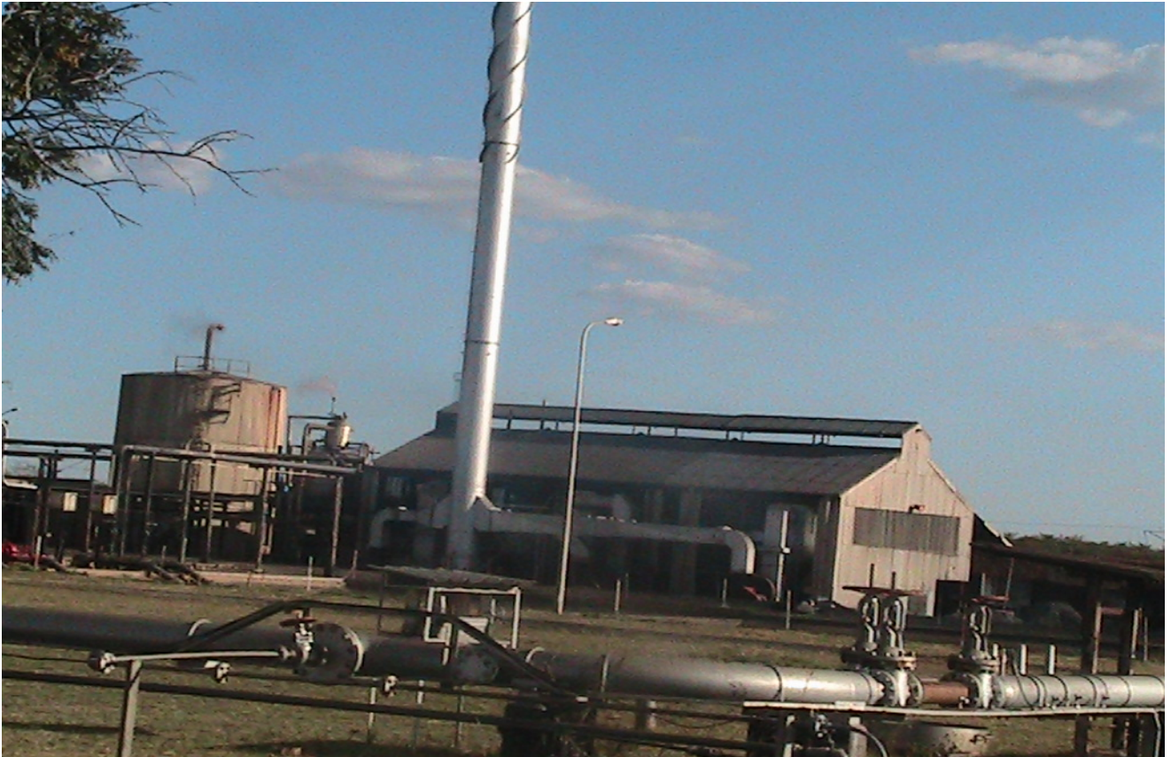
Figure 20: Boiler plant at S.C.I Date taken: 24 Sept 2012
