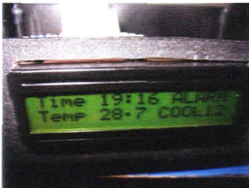
Figure 3.9: The temperature of the controller measured the same as DrDAQ
