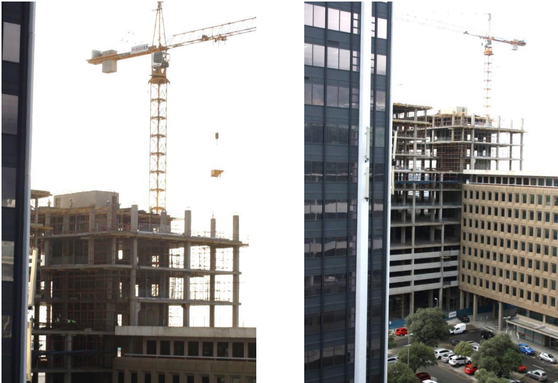
Plate 5.4: Close proximity of construction to existing buildings (Christiaan Barnard Hospital, Cape Town Urban Centre, April 2015)
