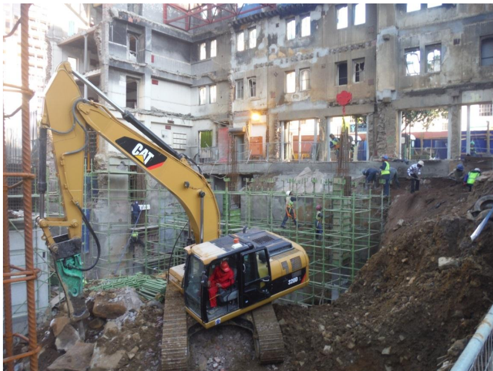
Plate 5.5: Restricted space and personnel in close proximity to machinery (Touchstone Office Development, Cape Town Urban Centre, August 2013)
