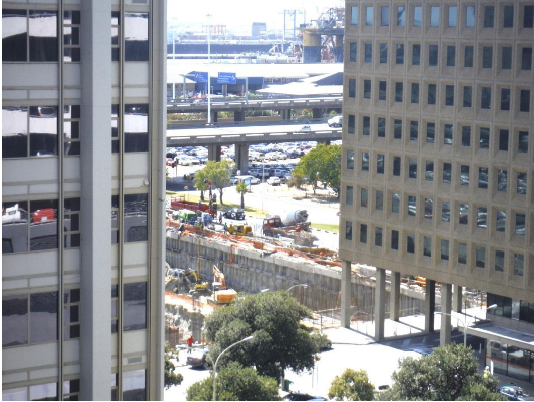
Plate 5.3: Close proximity of construction to existing buildings (Christiaan Barnard Hospital, Cape Town Urban Centre, March 2014)
