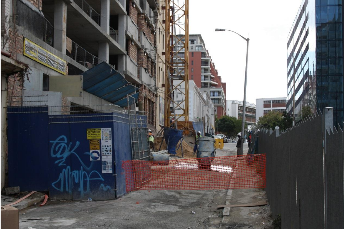
Plate 5.7: Construction materials and storage containers spill into the adjacent street necessitating road closure (Touchstone Office Development, Cape Town Urban Centre, April 2015)
