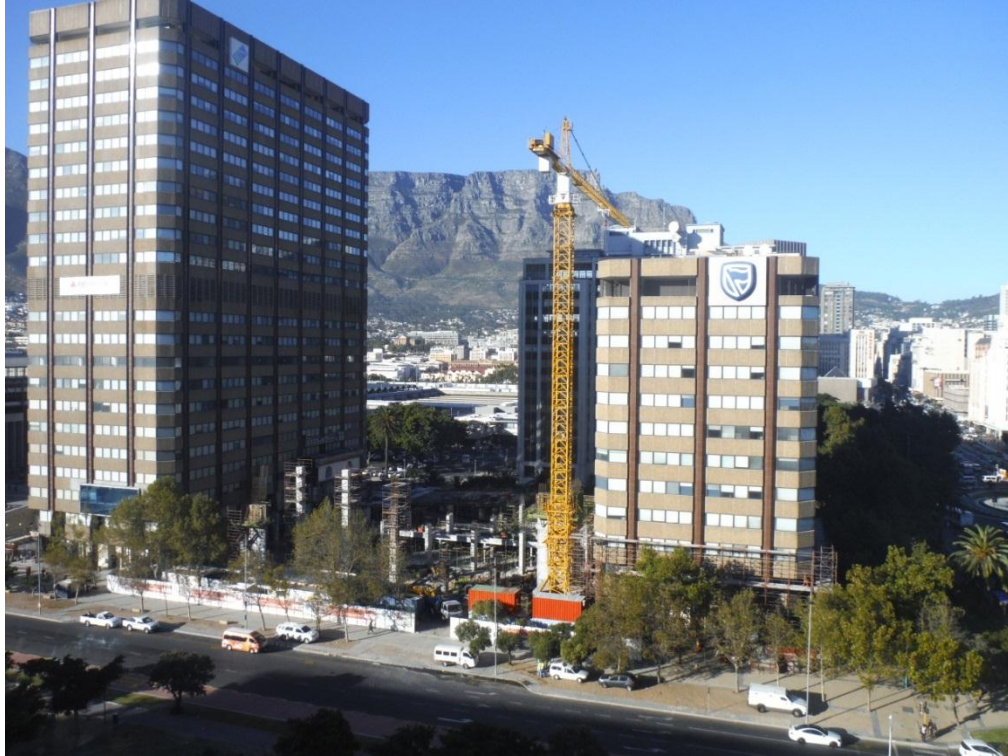
Plate 5.11: The confined site and limited access has required intricate planning of the positions of cranes and site operations (The Towers, Cape Town Urban Centre, March 2013)
