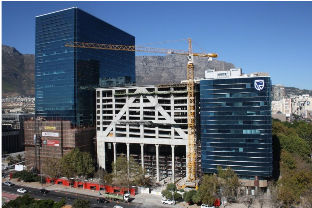
Plate 5.12: The use of BIM technology has allowed the modelling of the layout to ensure clashes are limited and interference with existing buildings and foundations avoided (The Towers, Cape Town Urban Centre, April 2015)
