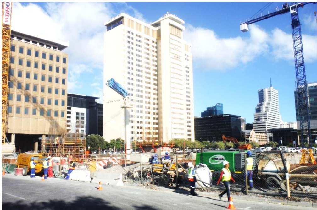
Plate 5.2: The safe movement of material, damage to materials and location of materials (Christiaan Barnard Hospital, Cape Town Urban Centre, 2014)
