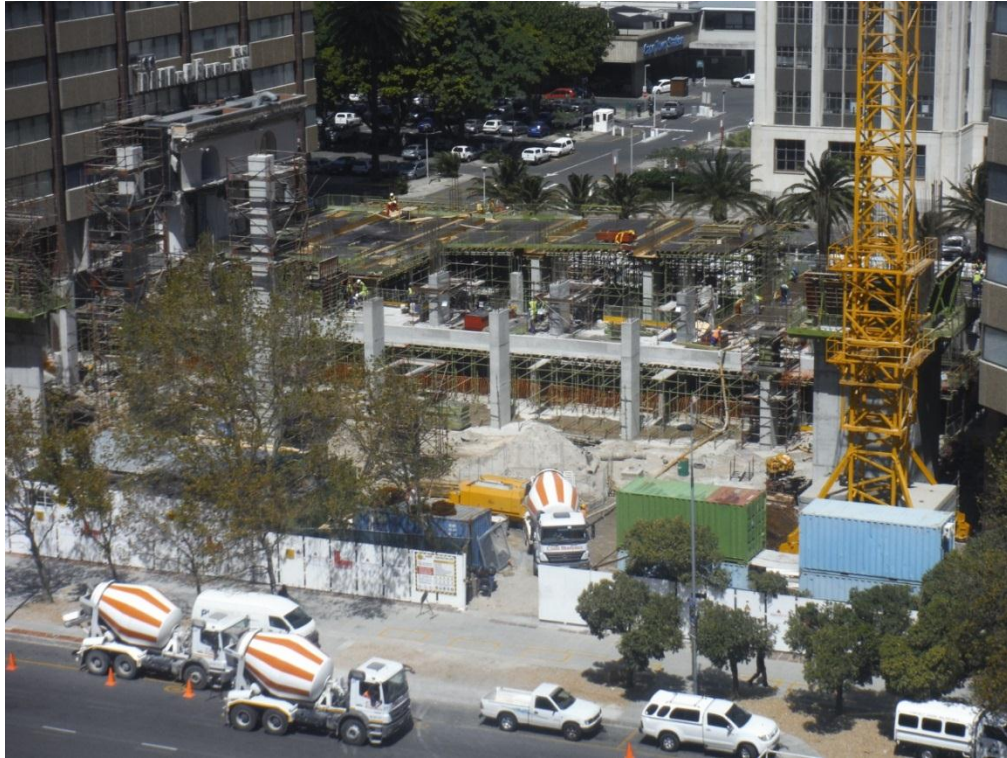
Plate 5.13: The first phase of the project was the demolition of an existing four-story building above a basement that continues to operate as a parking garage with active traffic movement (The Towers, Cape Town Urban Centre, March 2013)
