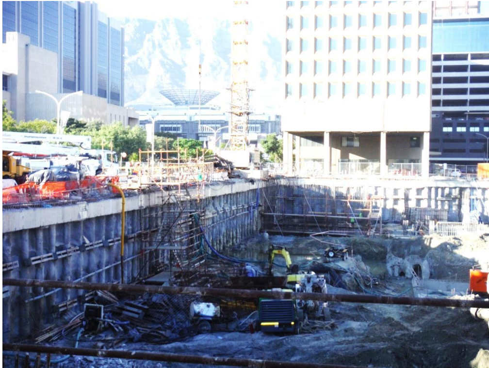
Plate 5.1: Confined space, congestion and restricted access for delivery of materials (Christiaan Barnard Hospital, Cape Town Urban Centre, 2014)
