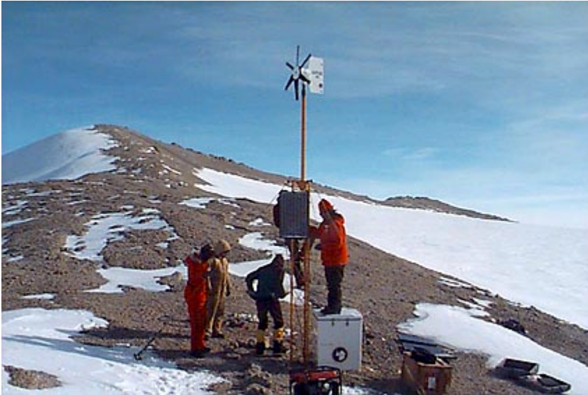
Figure 2.19: Wind Turbine Powered Telecommunication Station
