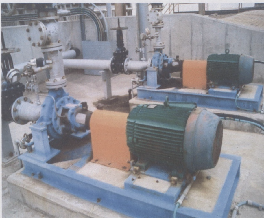
Figure 6.1 Pump drive in a petroleum refinery
