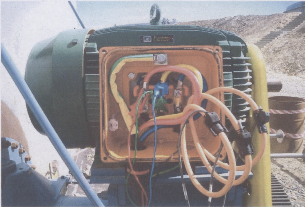
Figure 4.4 Current transformers connected to a HE-motor during a motor test
