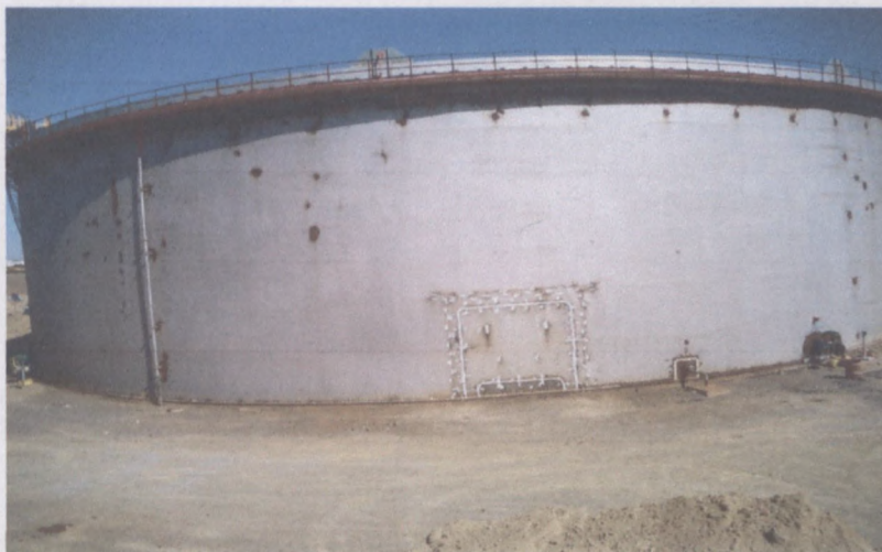
Figure 3.2 Petroleum storage tank
