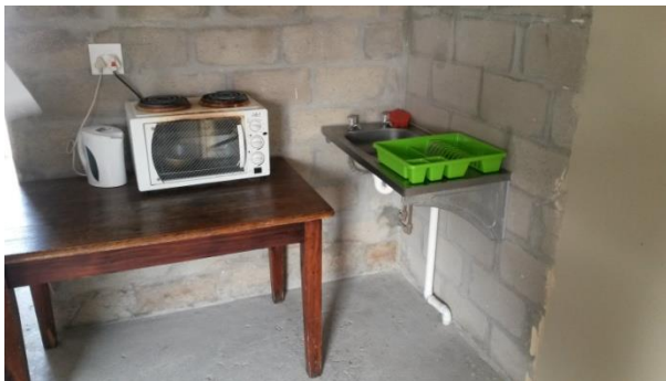
Onsite Image 68: Installation of the kitchen area without any wall surface treatment.
