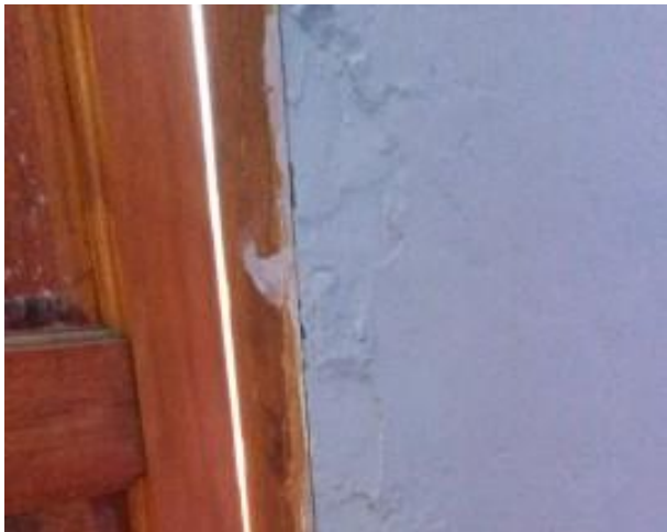
Onsite Image 34: Door installation that was poorly constructed and continually failing.
