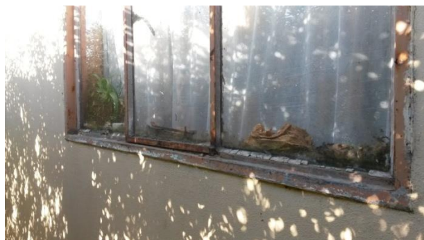
Onsite Image 44: The windows that were installed with the construction of the house are starting to fail.
