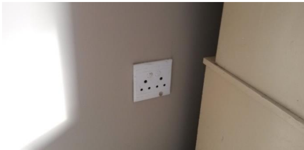
Onsite Image 67: Houses are fitted with electrical points internally.
