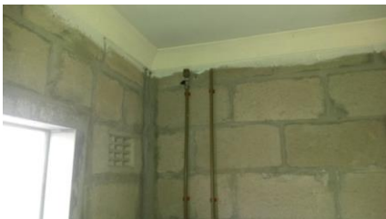
Onsite Image 17: Exposed piping that is assumed to be connected to the geyser, although this has not been installed, even though it is part of the building contract
