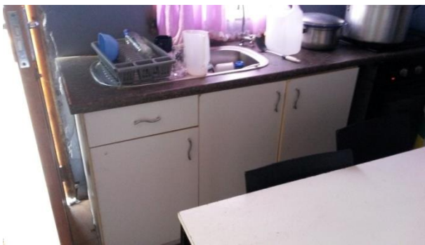
Onsite Image 37: Internal kitchen space with little manoeuvring space and with all the plumbing installed by the residents.
