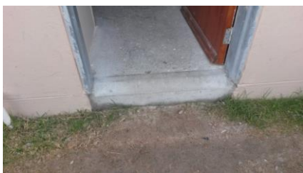
Onsite Image 13: Stepped access at the entrance to a house, which has a rise of more than 170mm; this does not comply with SANS 10400 Part S of 2011
