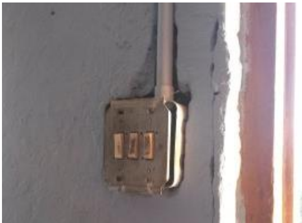
Onsite Image 35: Electrical wiring that was residents have installed.
