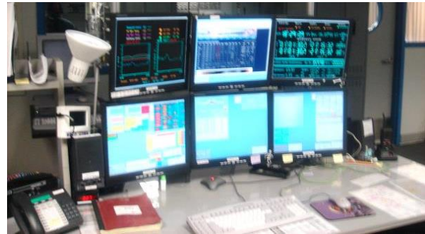
Figure 2.7, Keck HQ Control Room Smith, 2012
