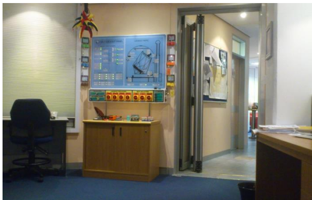
Figure 4.6, Telescope Lock-out Panel in the Control Room (Author, 2015)
