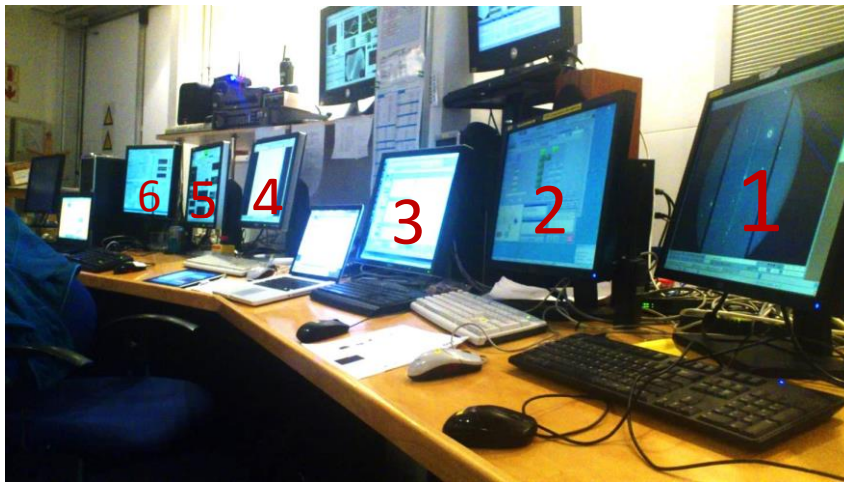
Figure 4.5, Inside the Control Room (Author, 2015)
