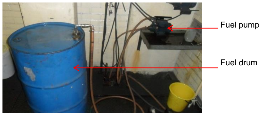
Figure 3.3: 1st room with fuel and fuel pump
