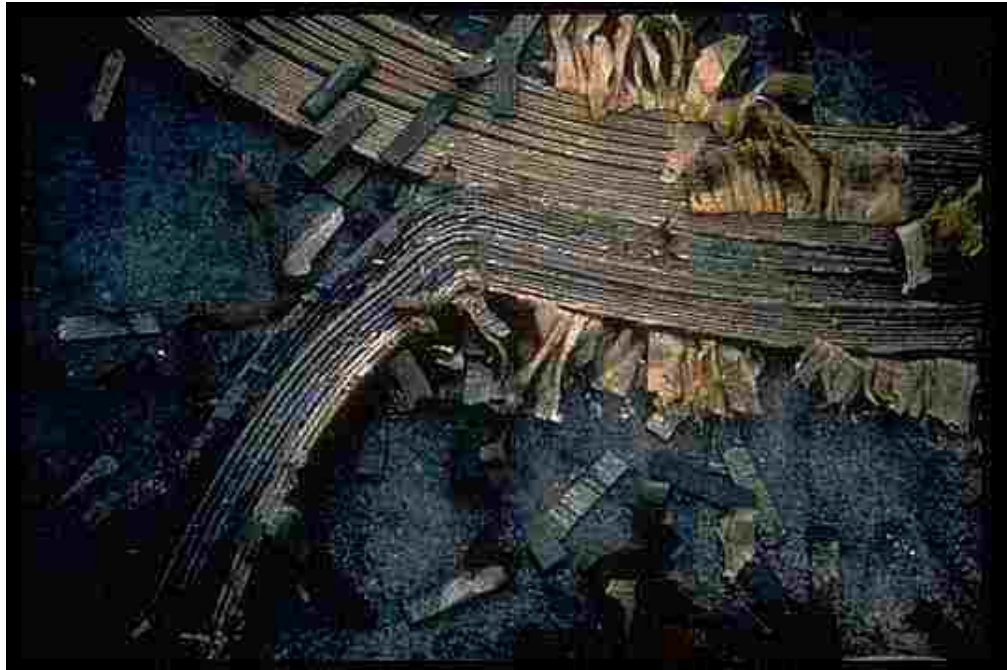
Figure 2.14: Effects of transformer heating associated with GIC. Adopted from http://www.spaceweather.gc.ca/tech/se-pow-eng.php .
