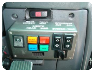
FIGURE 4.10: SWITCH CONTROL BOX
