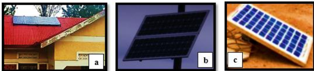
Figure 4.1: Some PV panel installations in sub-Saharan Africa: a) Mounting on a 29^\circ roof at the equator in Uganda; b) Mounting at 50^\circ in Cape Town, South Africa; c) Starter panel unit near the equator in Kenya.
