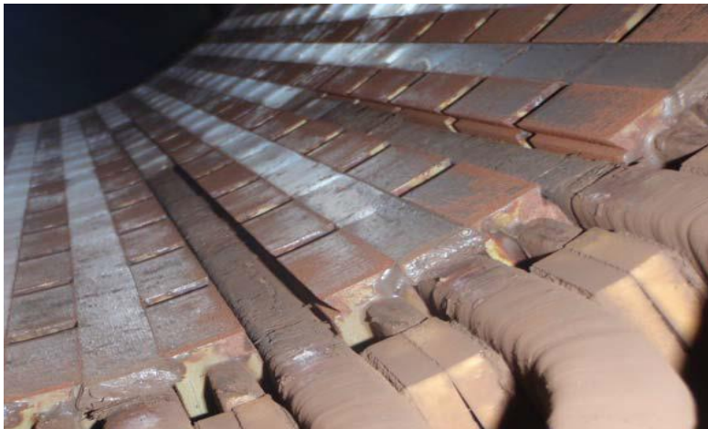
Figure 27: Missing stator slot wedges
