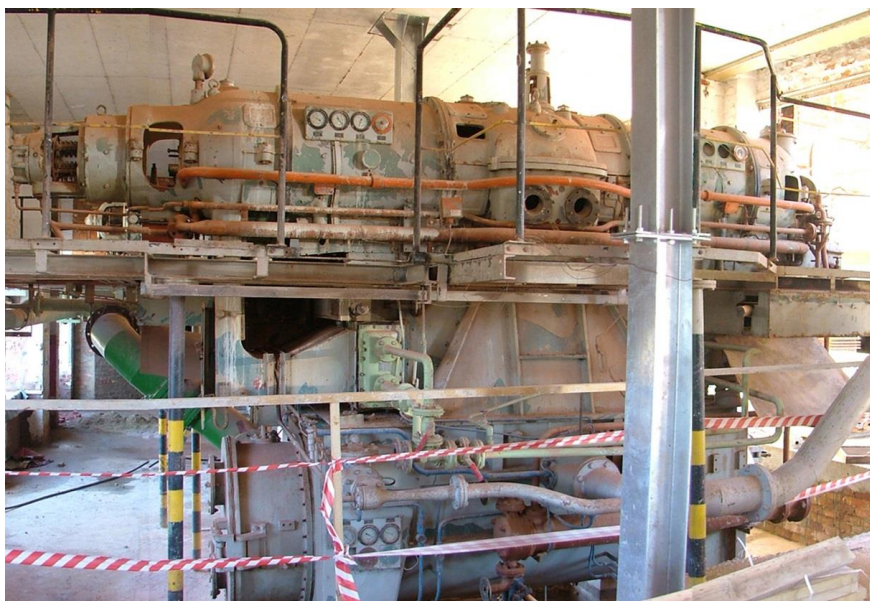
Figure 4-33: A further view of the turbine hall before reuse (source: Louw, no date)
