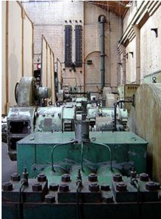
Figure 2-23: View of retained power station machinery at the Wapping Project (source: www.bluebadgestyle.com )
