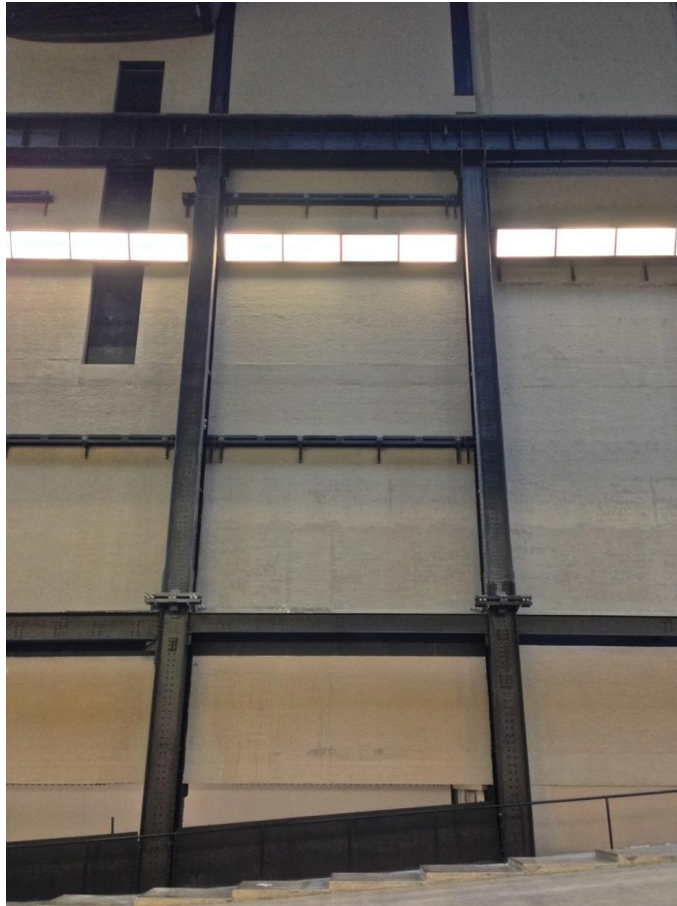
Figure 2-19: Interior of the Tate Modern's Turbine Hall showing exposed original steel framing (source: researcher's own)
