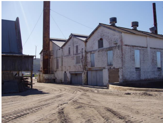
Figure 4-3: Western elevation of the Thesen Island power station before reuse (source: Louw, no date)
