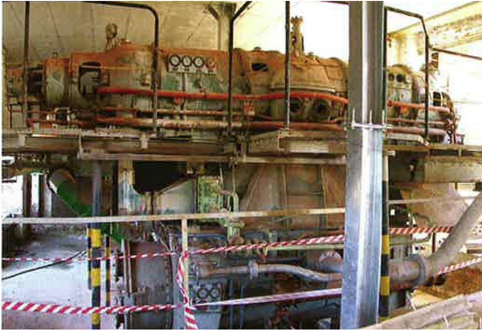
Figure 4-44: Before: the turbines in their dilapidated state before reconditioning (source: Architecture SA, 2011)
