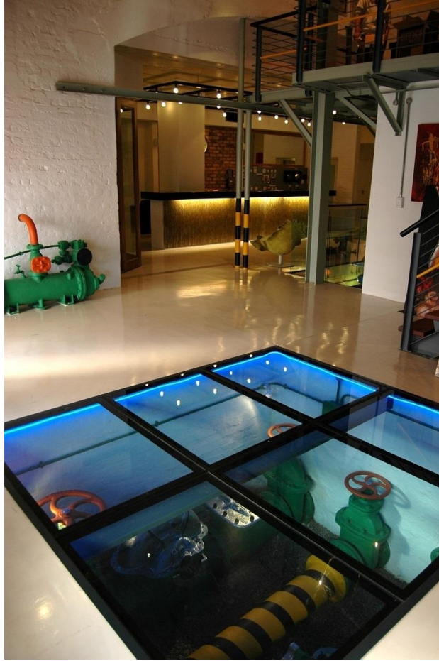
Figure 4-37: Reception area showing machinery placement, including the walkable glass floor with below surface machinery (source: Architecture SA, 2011)
