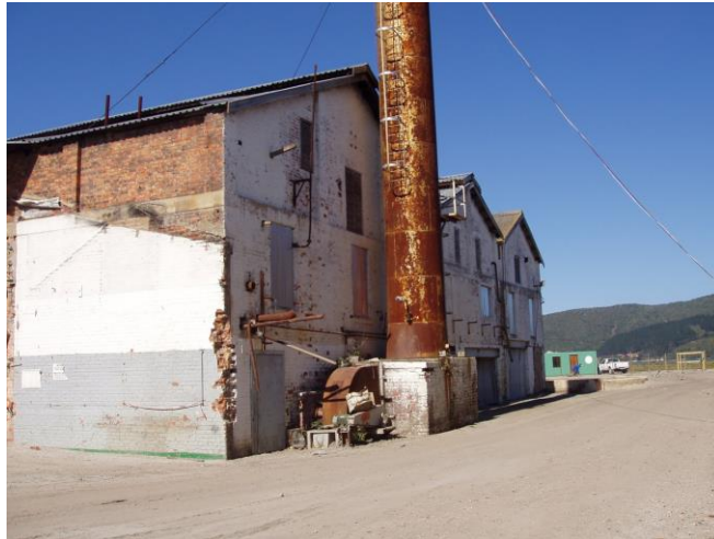
Figure 4-2: Western elevation of the Thesen Island Power Station before reuse (source: Louw, no date)
