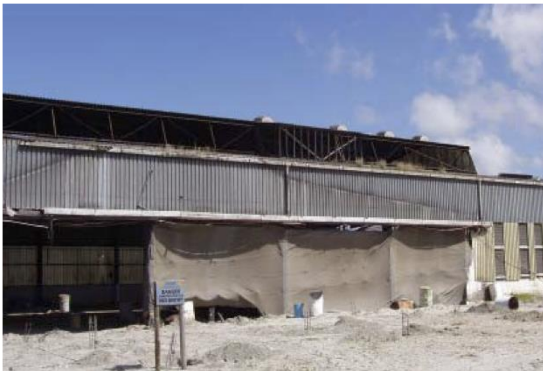
The dilapidated Parking Shed before adaptive reuse (source: Urban Futures, 2008)
