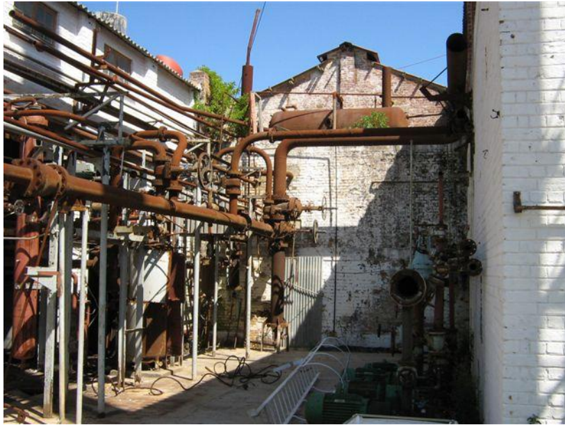
Figure 4-26: View of the ‘courtyard before adaptive reuse showing extensive piping (source: Louw, circa 1998)
