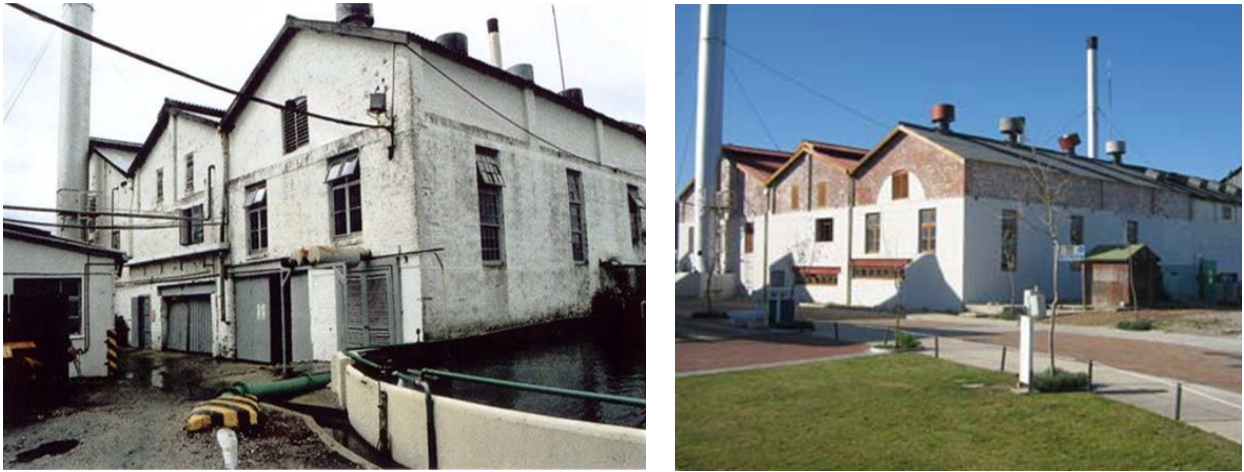
Figure 4-13: The Thesen Island power station before and after initial preservatory works (source: Louw, no date)
