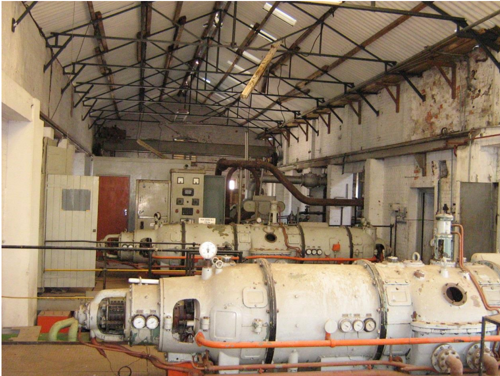
Figure 4-32: The turbines in the power station before reuse (source: Louw, no date)
