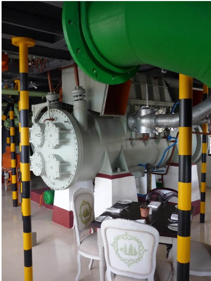
Figure 4-41: Further view of repainted turbine in the dining area (source: researchers own, 2012)
