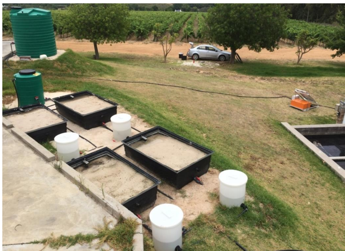
Figure 3.6 A picture of the installed BSF system on site: anti-clockwise from top right: solar pump, 5000 L holding tank, 500 L tank and four filter modules with flow control tanks
