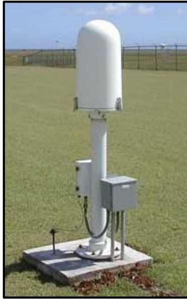
Figure 2.15: Ground-based lightning sensor for detection of electromagnetic radiation from lightning
