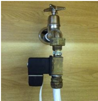
Figure 4.13 Solenoid valve connected to inlet pipe of geysers to control the water into the geysers
