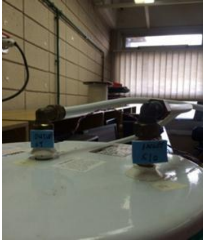
Figure 4.12 Two LM35 temperature sensors on inlet and outlet pipes
