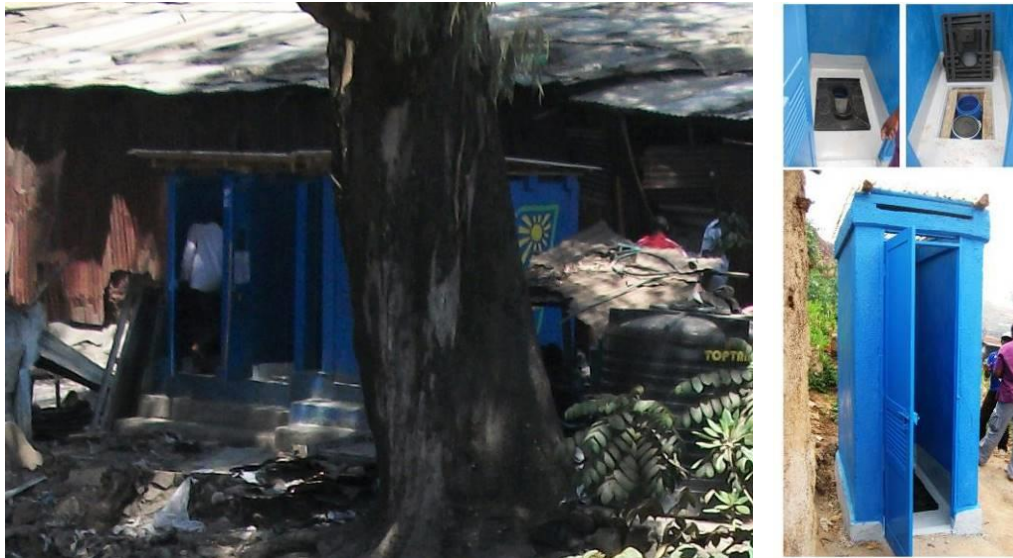
Figure 4.15: Composting toilets in Gikomba Market, Nairobi; and an inset of working components
