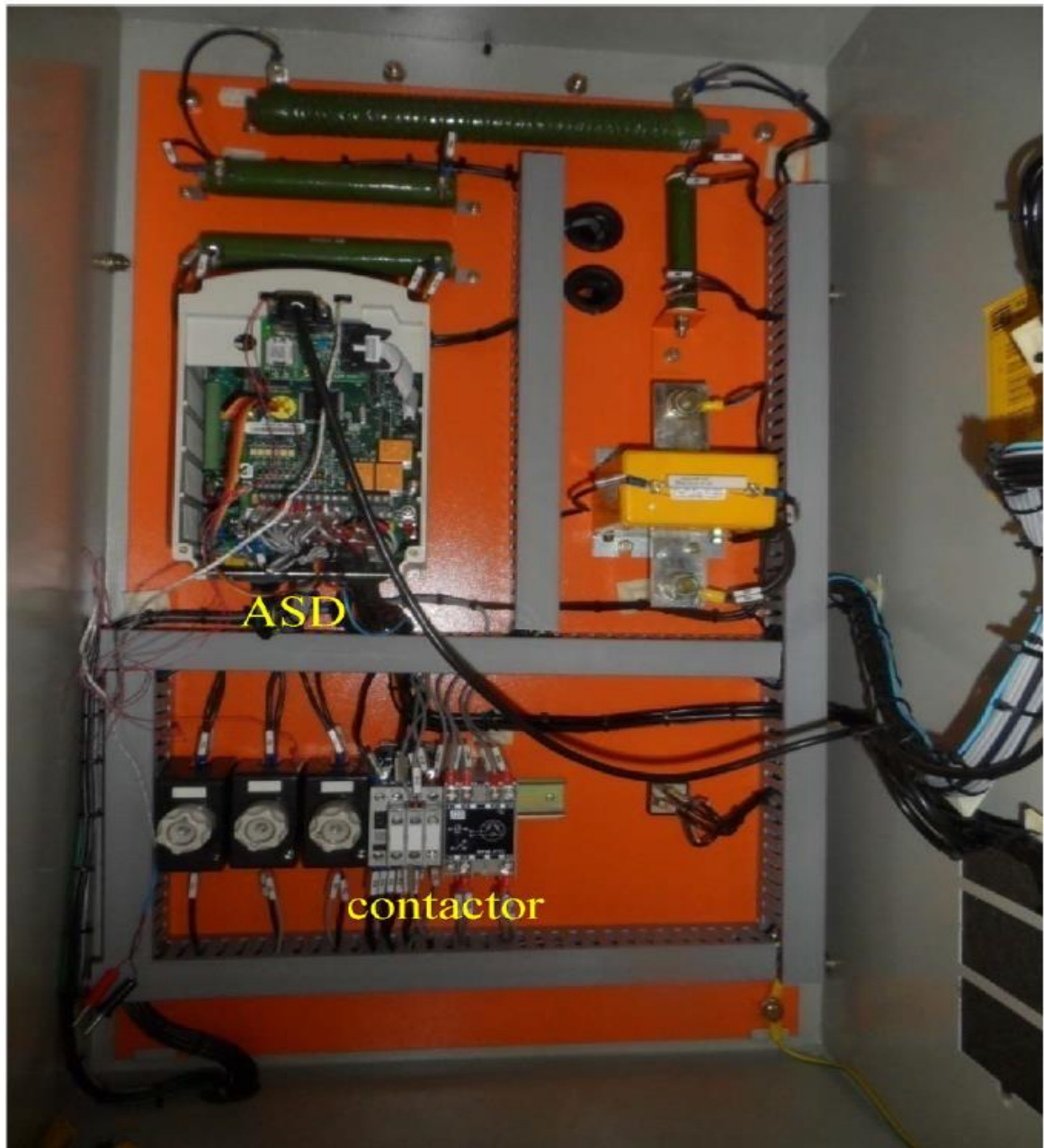
Figure 3.9: Interior of the test control panel with an ASD and induction motor
