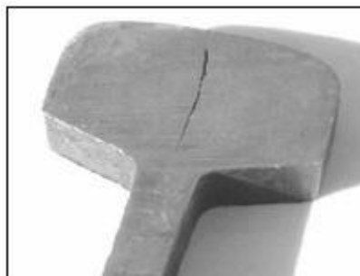
Figure 2.7: Longitudinal vertical crack [Granstrom, LTU]
