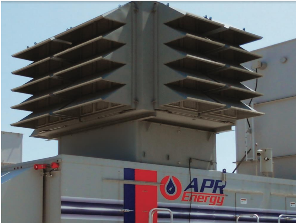
Figure 3.2: Inlet air of APR gas turbine (APR, E., FT8)
