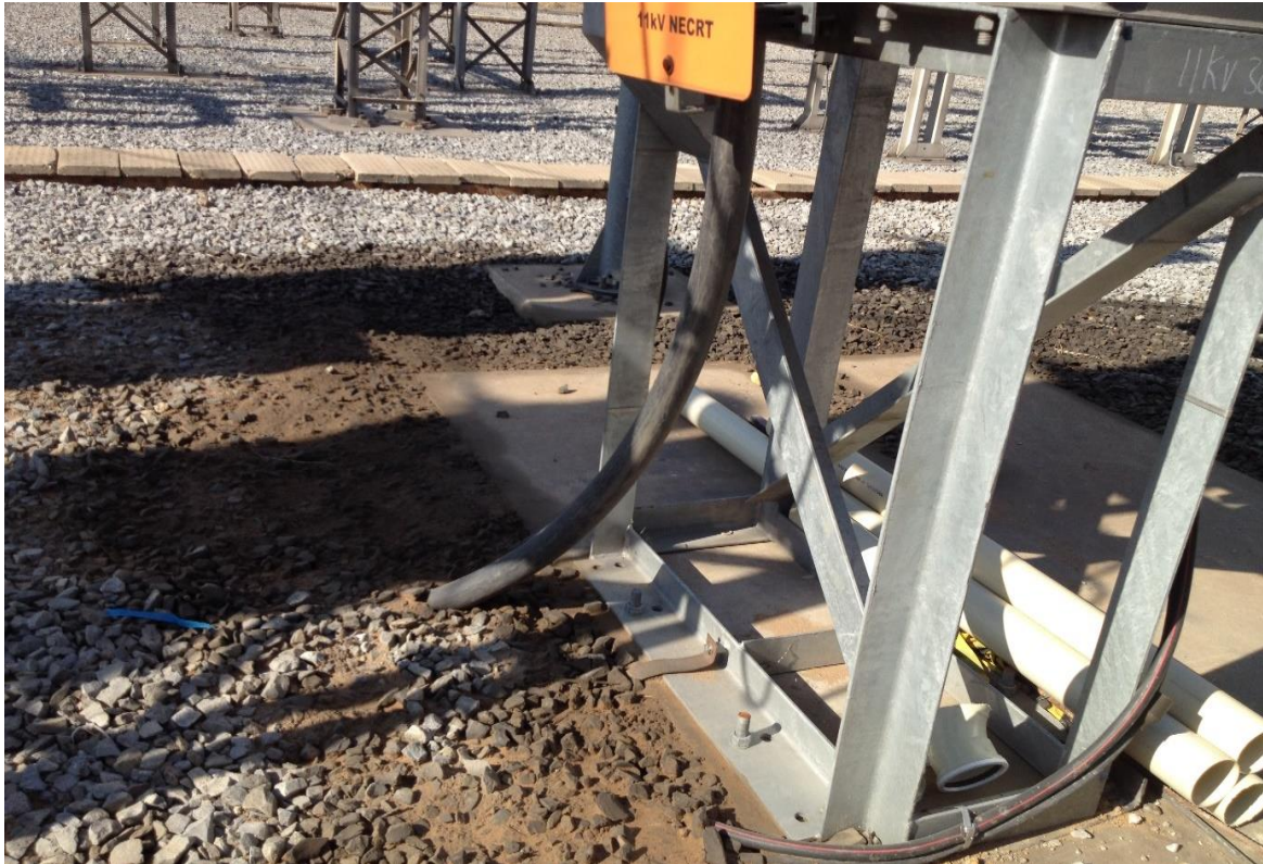
Figure 4. 22: Land pollution from exploded NEC Transformer
