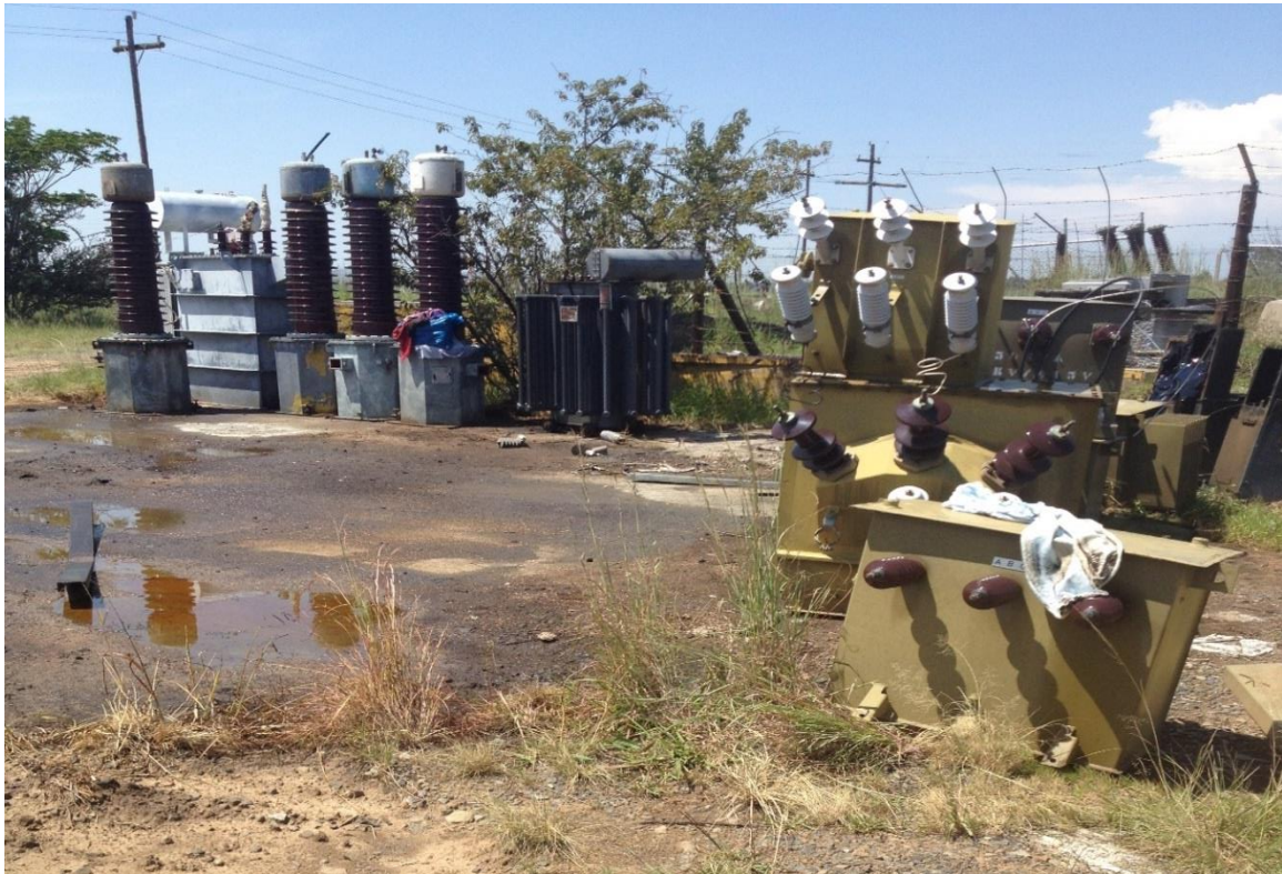
Figure 4. 19: Oil spill at the storage area
