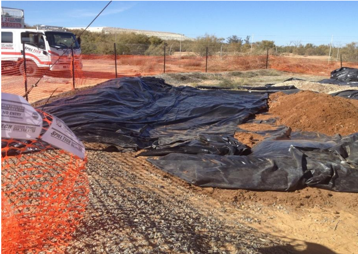
Figure 4. 20: Contractor cleaning up oil spill
