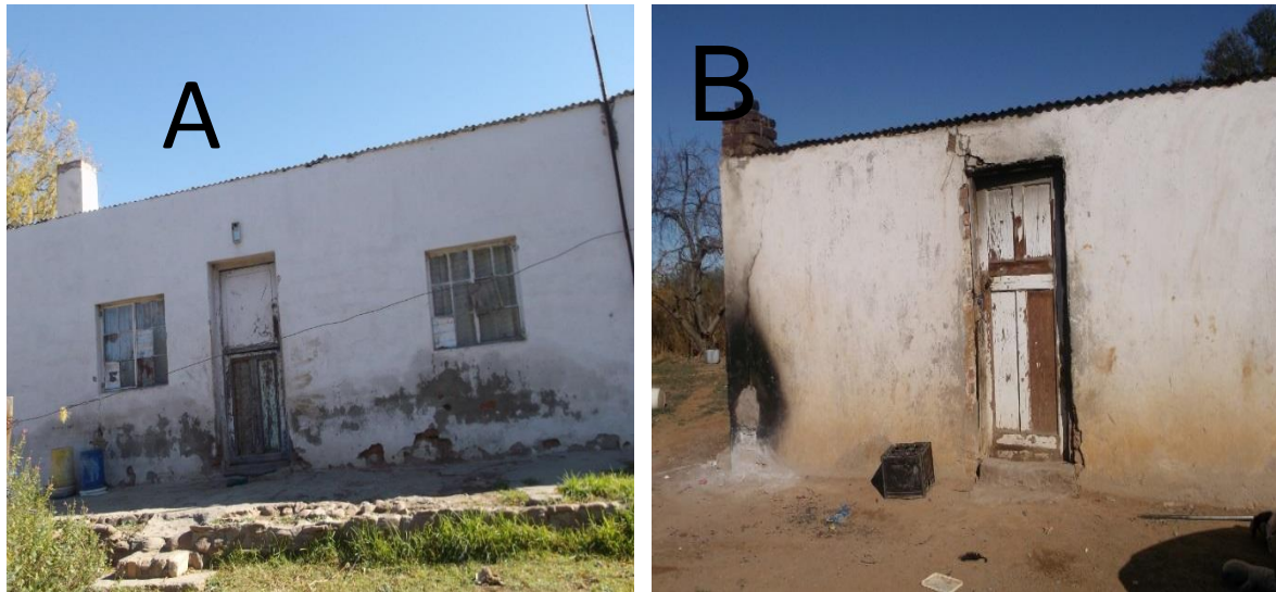
Figure 6.4: The dilapidated condition of the farm workers' houses in Cradock farms.
