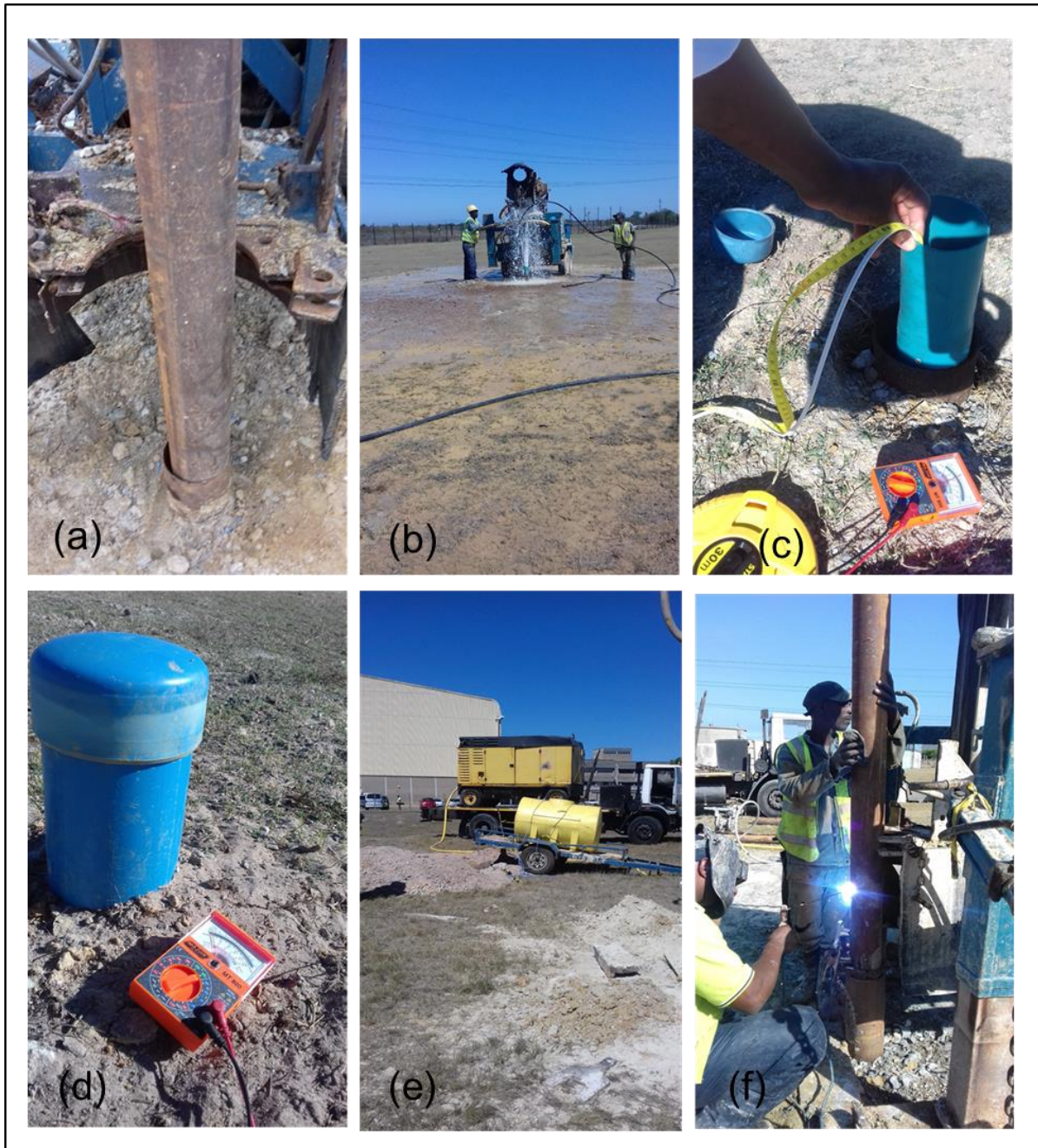
Figure 3.2. Borehole construction: (a) drilling inside casing, (b) borehole pressurisation, (c) water depth quantification, (d) bore-hole closing, (e) generator to pressurise groundwater and (f) welding a permanent casing.
