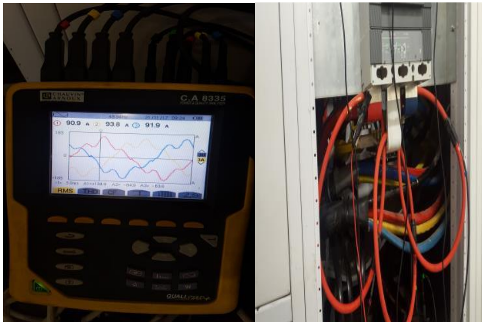
Figure 7.3: Illustrates PQ measurement instrument at langerberg mall 1.5MW grid-tied system
