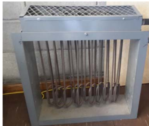
Figure 7-14: The resistive, high voltage, element bank used for initial load testing.
