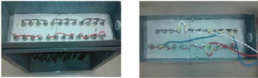
Figure 7-15: (a) The load resistances connected in parallel. (b) The phase resistances connected in a delta configuration.
