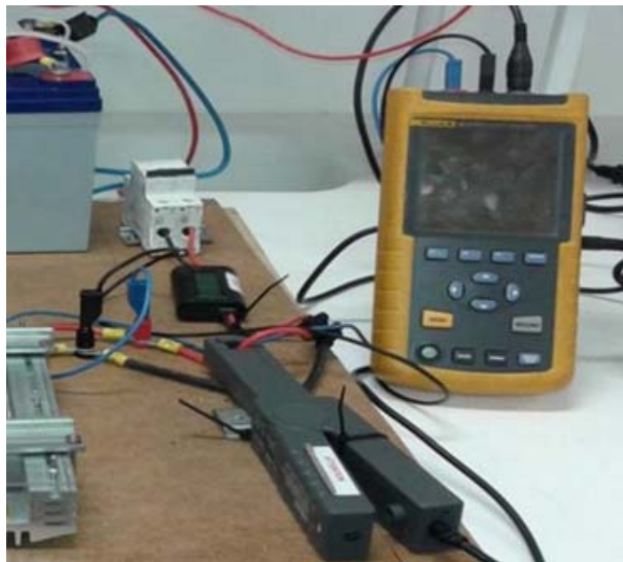
Figure 7-10: The input side to the motor drive together with the metering equipment.
