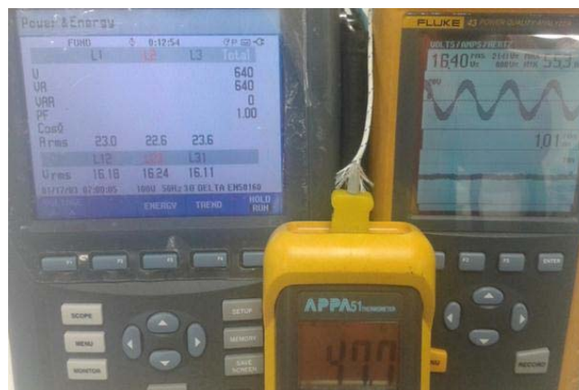
Figure 7-23: Maximum cable temperature reached when using the Fluke 435B on the Power and Energy display option.
