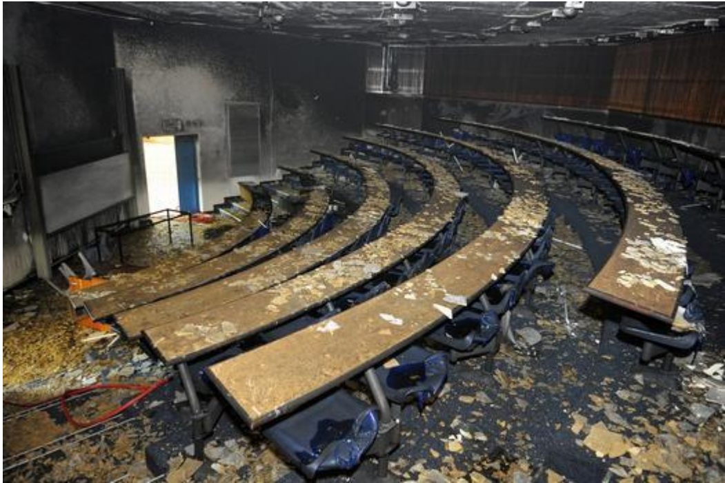
Figure 4.8: Damage done to classrooms (Ritchie, 2017)
